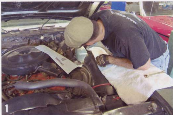
1 Using a line wrench on the rigid brake lines keeps the wrench from slipping off the brake line ferrules, rounding them off and causing other problems. A good set is a worthwhile investment.
