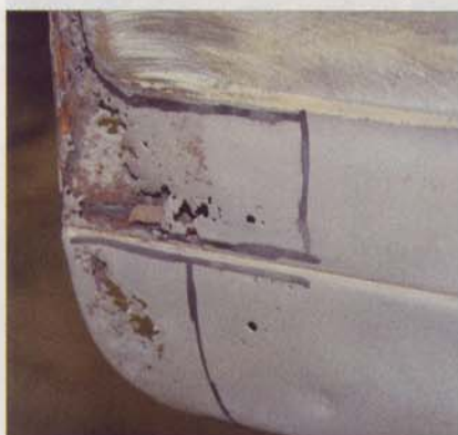
3 Cut lines are drawn on all cancerous areas. Jelinek was very conservative to remove the least amount of metal necessary.
