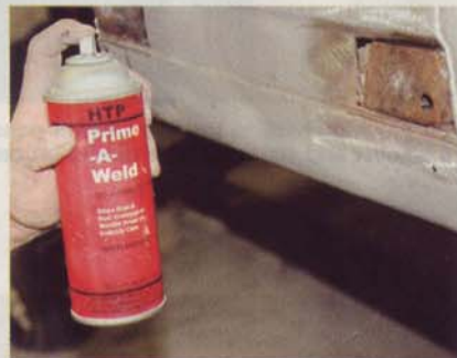
7 The panel and inner structure were ground clean before Jelinek sprayed HTP Prime-A-Weld, a weld-through primer, on the bare metal edges.
