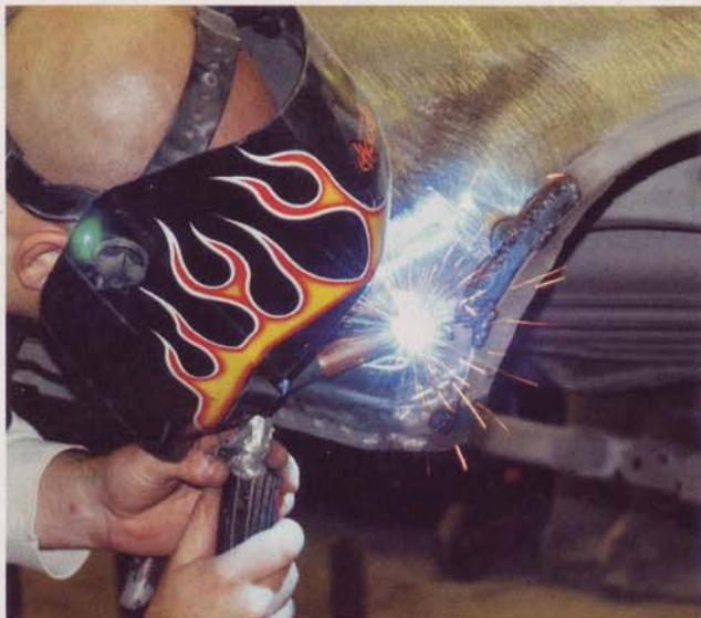
10 Moving back to the rear quarter-panel, Kevin Rock took over and continued the careful process of metal repair.
