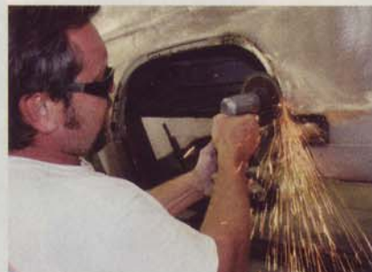
9 With the new panel in place, Jelinek used a 3M 24-grit 5-inch grinding disc to smooth the welds.
