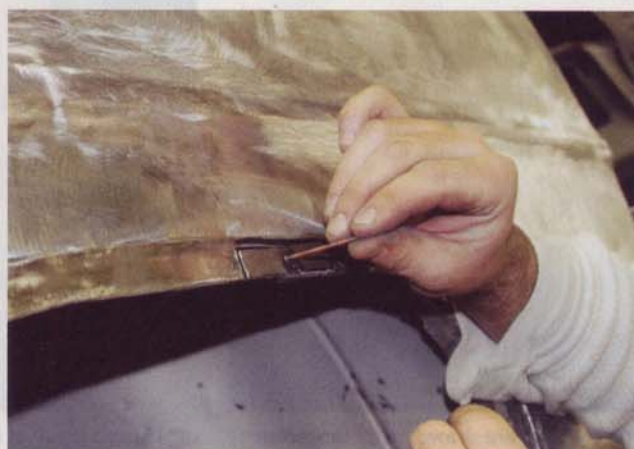
15 A small patch of metal is hard to handle, so Rock used a stud gun to attach a stud to the metal. By doing so, it can be held properly during welding.
